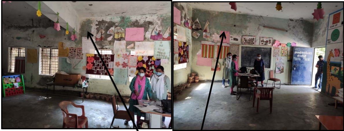
Faded paint, uneven walls
