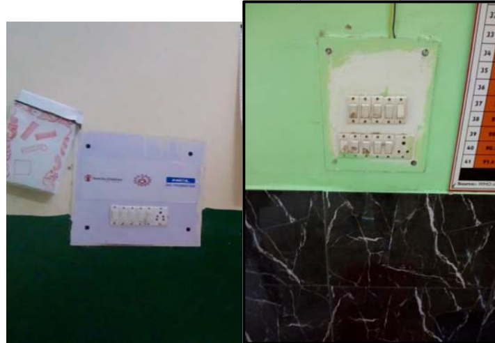
Switchboards at Chalera ChauraRaghunathpuram AWC No. 3
