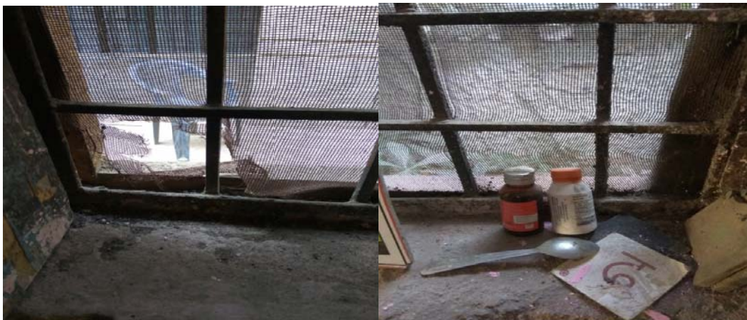
Windows covered with net and damaged at ChauraSahadatpur
