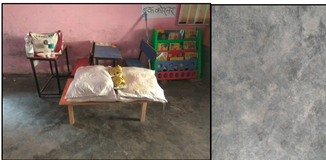
Cemented Flooring at ChauraSahadatpur, AWC No- 6
