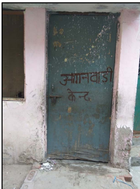
ChauraSahadatpur, AWC No- 6- Name written on the door of multi-purpose room
