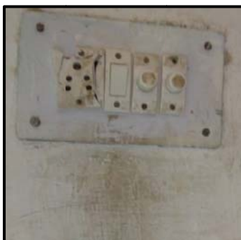
Switch boards at Rozayakubpur AWC No.1
